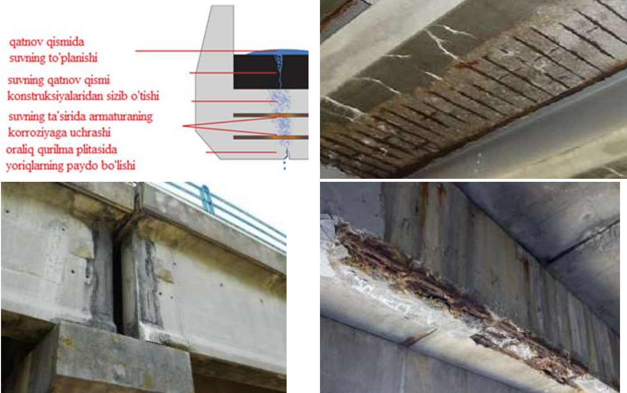
Figure 2. Defects caused by improper application of waterproofing.
