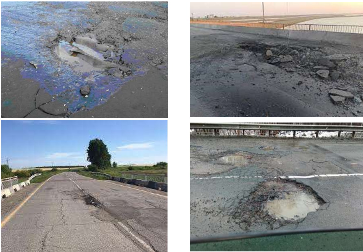
Figure 1. Different external effects as a result asphalt on the cover appearance to be defect and injuries
