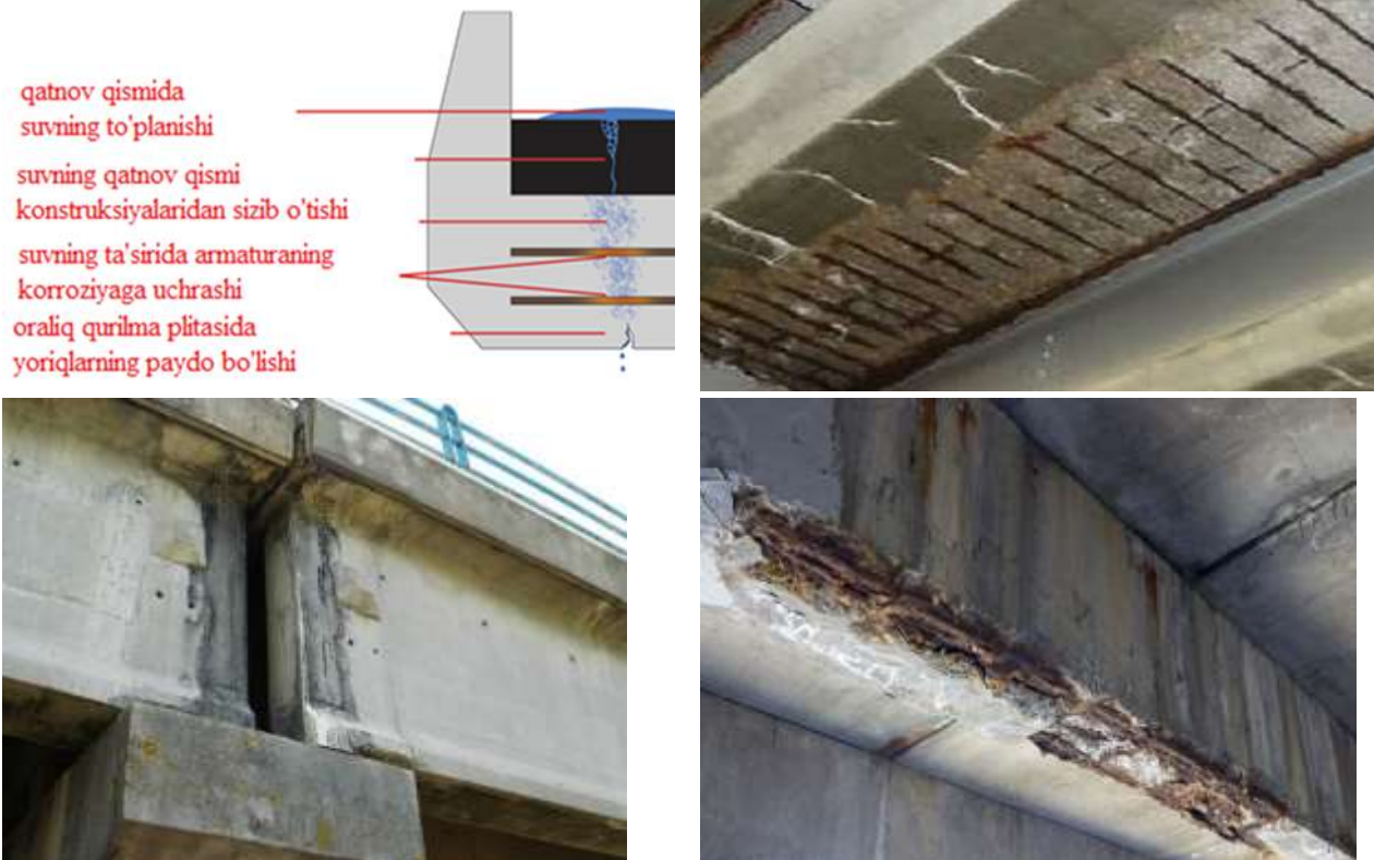
Figure 2. Defects caused by improper application of waterproofing.
